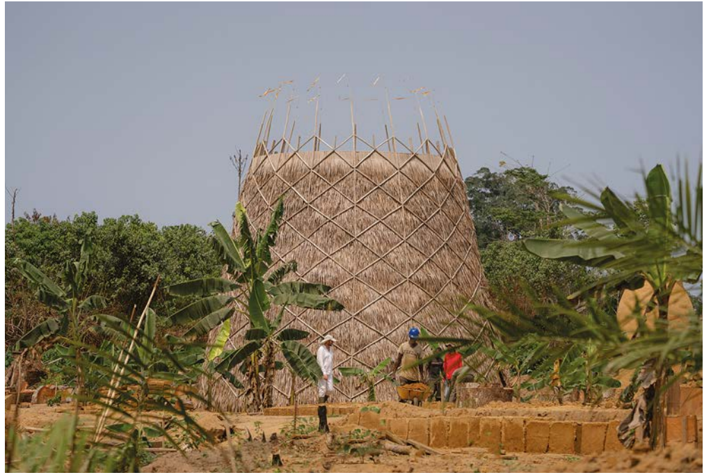
ABOVE: Built entirely from native materials and employing local labour, architect Arturo Vittori's Warka Village in Cameroon is a model for sensitive, community-driven development. Slated for completion in 2022, the project includes a bamboo and reed rain-harvesting tower (shown) that supports the sustainable enclave. PHOTO BY ARTURO VITTORI
