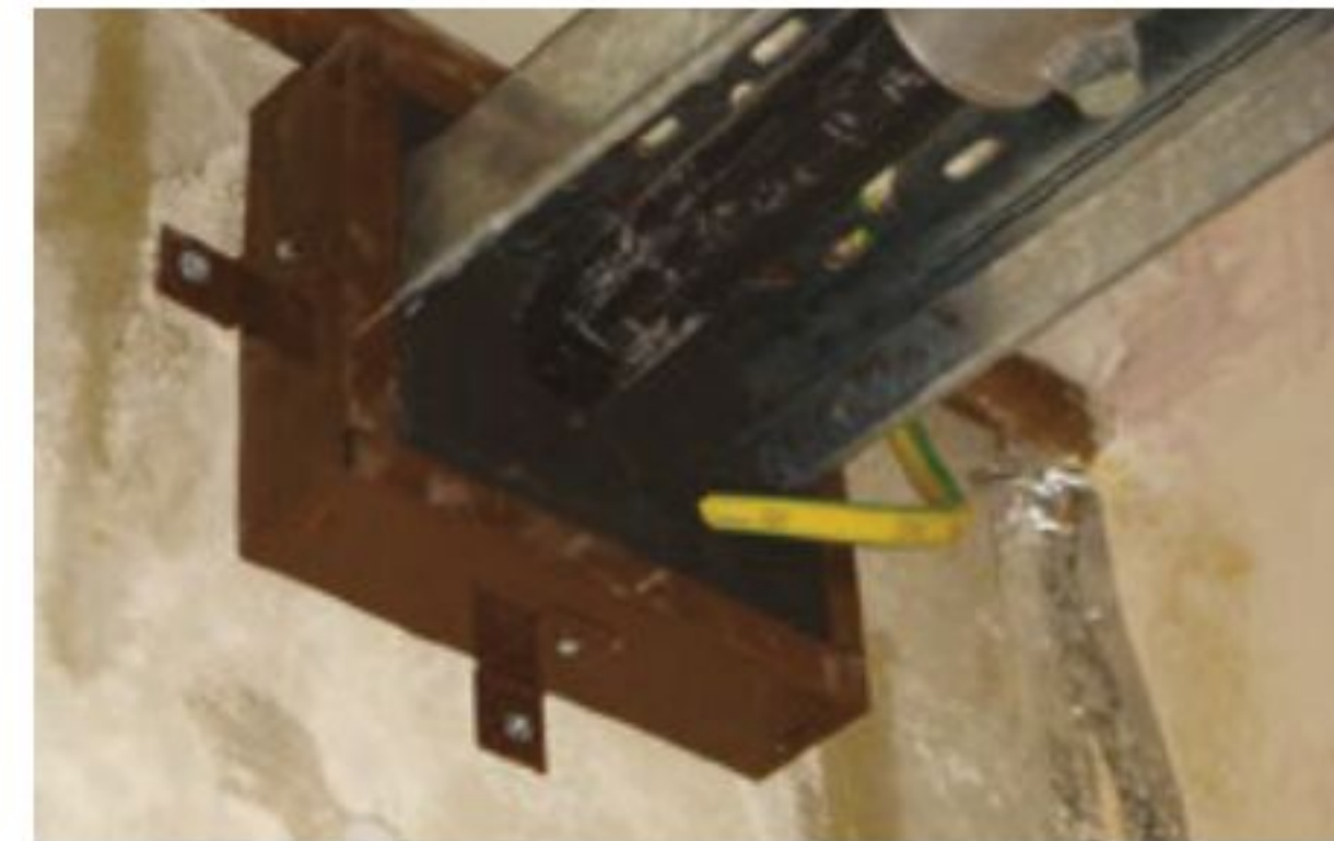
MULTI PURPOSE BOX BEING USED FOR DIFFERENT SERVICES
