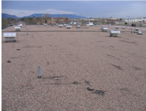
This was an old roof in need of resealing at Ft. Carson in Colorado. Photo courtesy of Neogard, a part of the Hempel group
