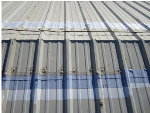
The surface must be exceedingly clean, and seams and penetrations must be properly prepared. Photo courtesy of Neogard, a part of the Hempel group
