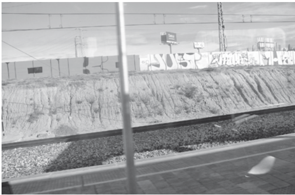
Figure 4.4. Steep eroded soil bank with parallel gullies and few plants. Eroded gullies in the silt and/or clay form and deepen mainly where plants are absent. Urban graffiti on wall. Madrid peri-urban area. R. Forman photo.
