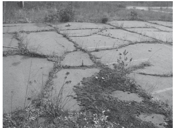
Figure 10.8. Plant succession on network of cracks of former parking lot. Short white lines indicated parking spaces; long parallel cracks indicate tarmac/asphalt strips originally put down; over time vegetation patches enlarge and interconnecting corridors widen. Sudbury in suburban Boston. R. Forman photo.
