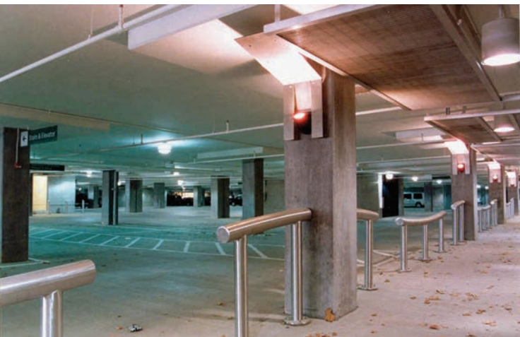
Separating pedestrian paths from vehicular circulation patterns to the fullest extent possible can reduce the chances that a vehicle will strike a pedestrian.
