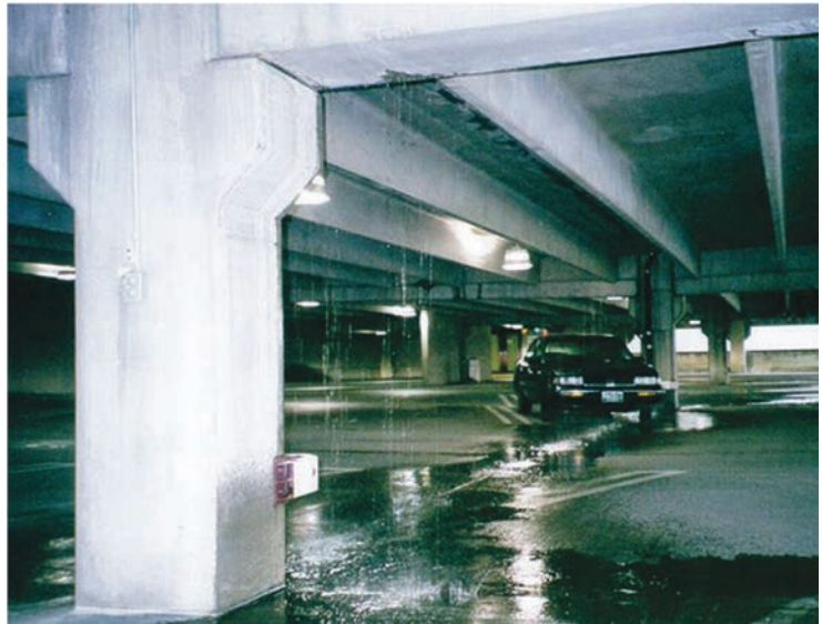
Water is a major causative agent in damage caused by corrosion and freezing and thawing.
