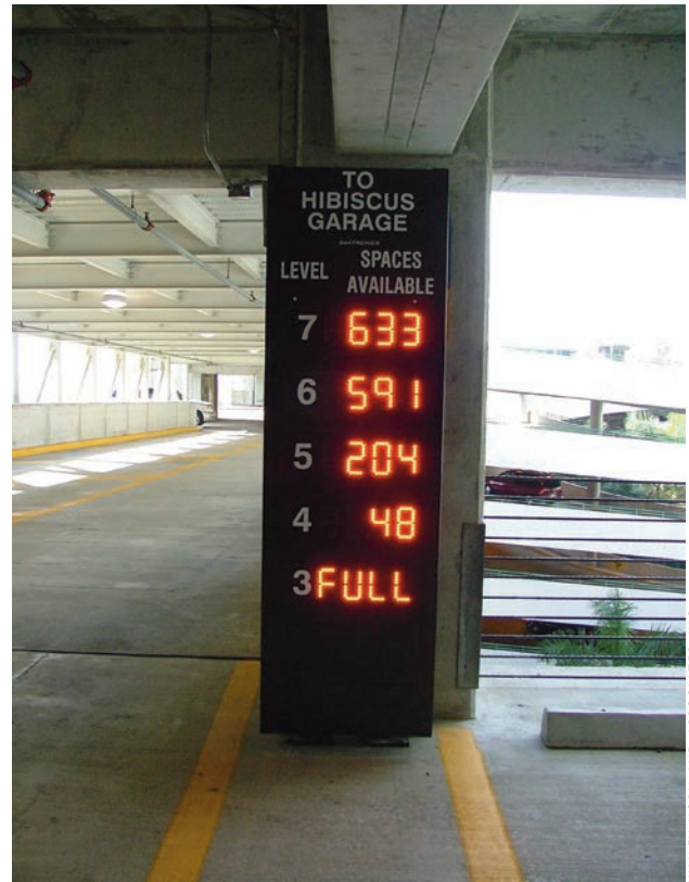
The parking structure at Fort Lauderdale-Hollywood International Airport, in Fort Lauderdale, Florida, employs a counting system that lets patrons know how many spaces are available on each level.
