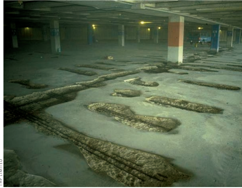
Patching a damaged floor slab can be expensive and cause lost revenue. Pictured here is a slab suffering from delaminations and spalls.
