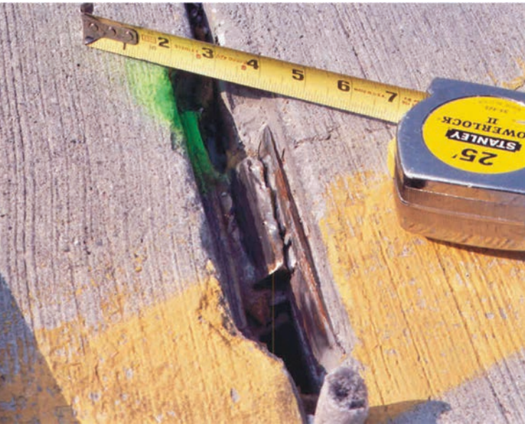
A failed tee-flange shear connector.
