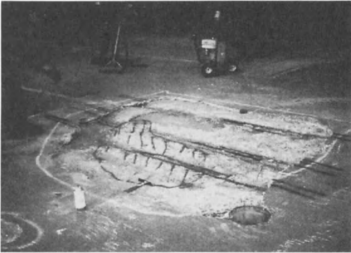
Figure 19-53: (a) Test well to observe condition of underlying substrate and reinforcement.
