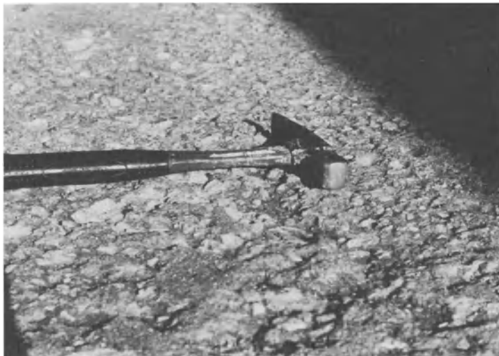
Figure 19-42 (c): Heavy scaling.
