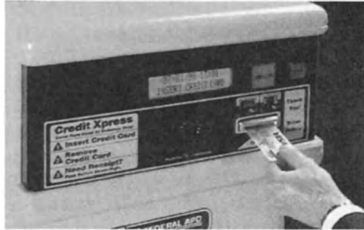
Figure 4-9. Credit card in/out at entry and exit lanes is becoming more common. Photo courtesy Federal APD.
