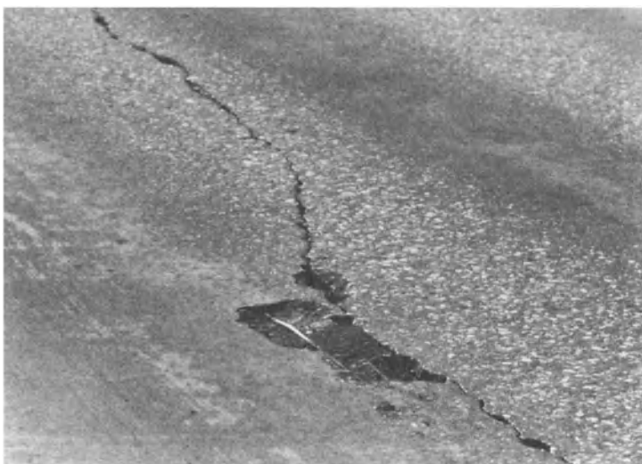
Figure 19-43: Surface abrasion and cracking.
