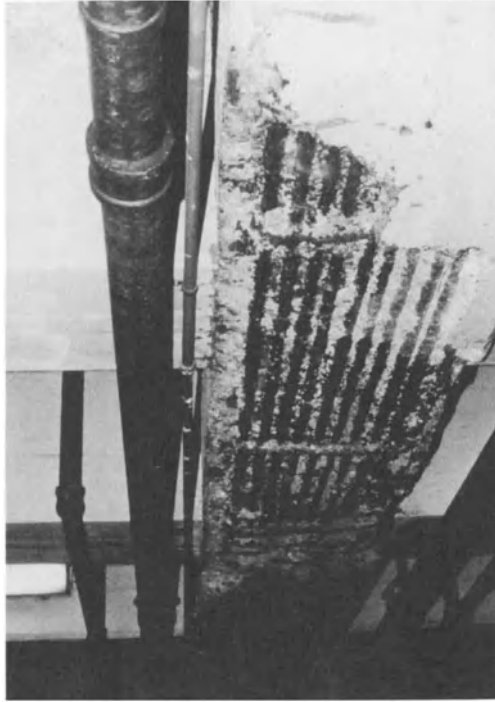
Figure 19-19(a): Concrete deterioration due to water leakage through slab crack.
