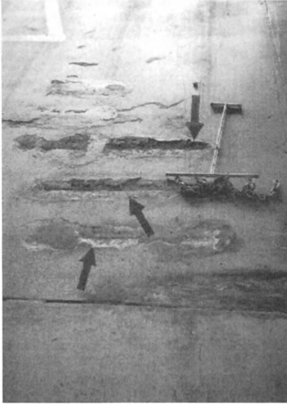
Figure 19-11: Shallow concrete cover will reduce “time-to-corrosion” of embedded reinforcement.
