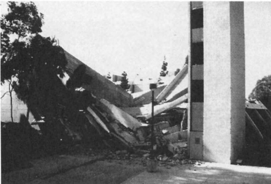
Figure 14-3: Complete collapse of a 3-story post-tensioned parking facility, Northridge, CA. (Photographs by S. K. Ghosh and Associates, inc.)
