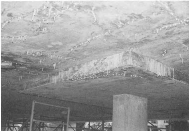
Figure 19-41: Leaching and formation of stalactite on underside of slab.
