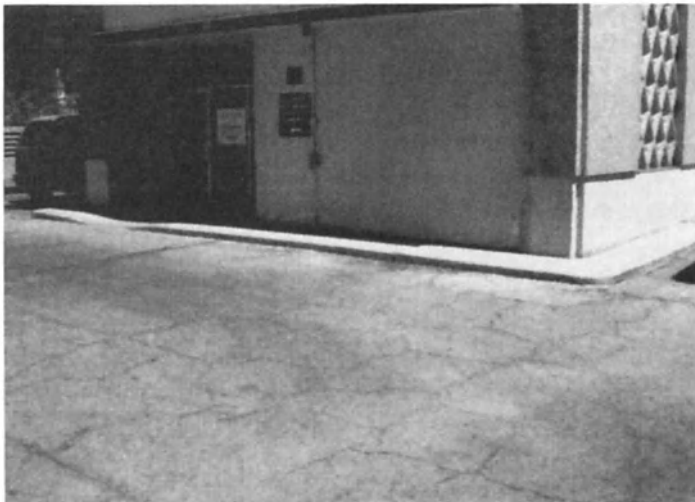
Figure 13-13: Protected membrane with asphalt overlay that needs replacement. The asphalt is extensively cracked and deteriorated by natural weathering.
