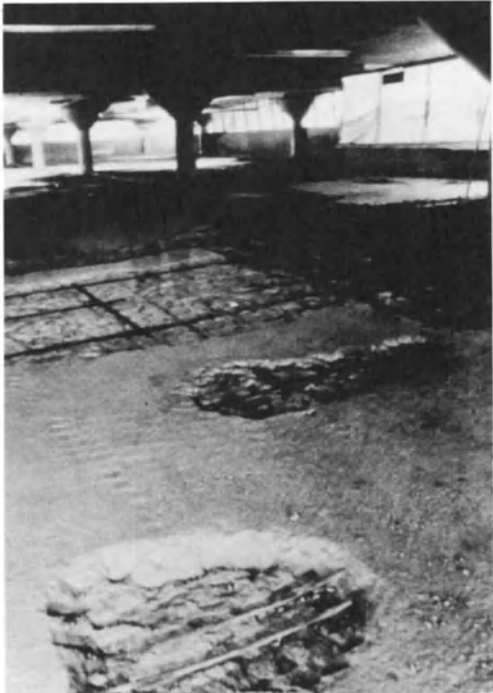
Figure 19-6: (a) Extensive concrete deterioration can adversely affect load carrying capacity of structural members.
