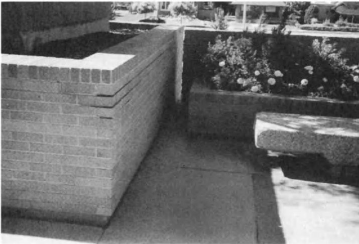
Figure 13-1 (contd.): (c) Protected membrane system driveway over parking garage. (d) Plaza deck planters.
