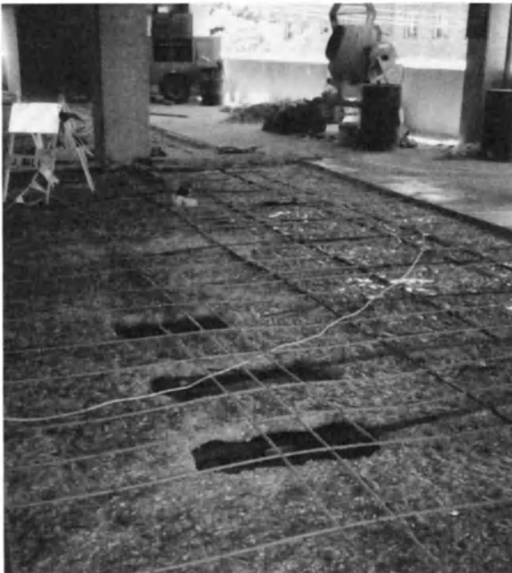
Figure 20-33(b): Strip patch repair showing removal of all top slab reinforcement over beam.
