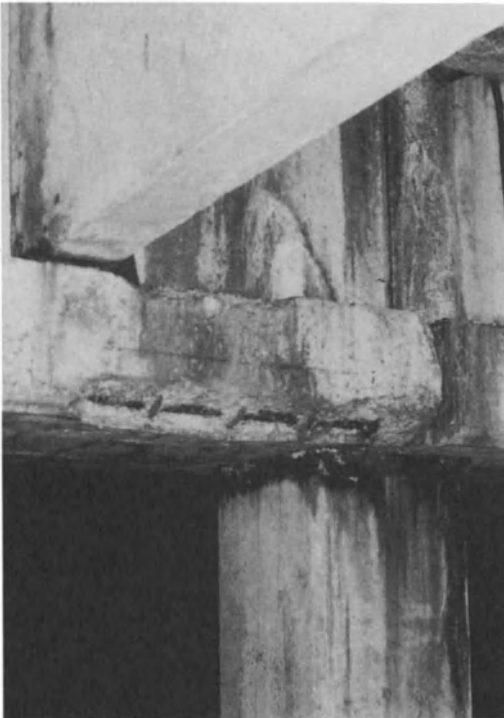
Figure 19-7: Corrosion of embedded reinforcement due to leaching and carbonation of poor quality concrete.
