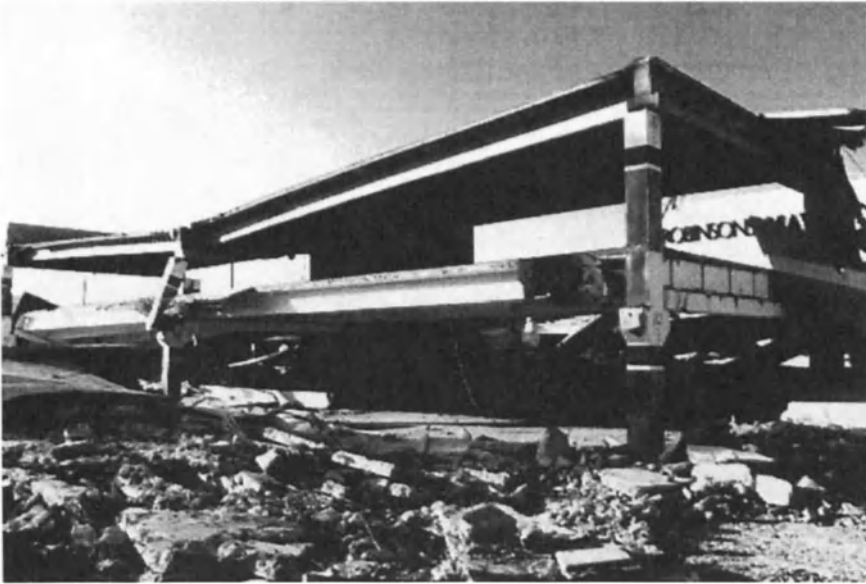
Figure 14-2: Complete collapse of a 3-story precast parking facility, Northridge, CA. (Photographs by S. K. Ghosh and Associates, inc.)
