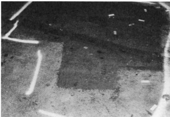
Figure 20-31: Delamination due to continuing corrosion within and beyond patch boundaries.
