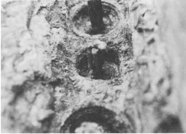
Figure 19-21(c) Corrosion of unbonded strand at end anchorage.
