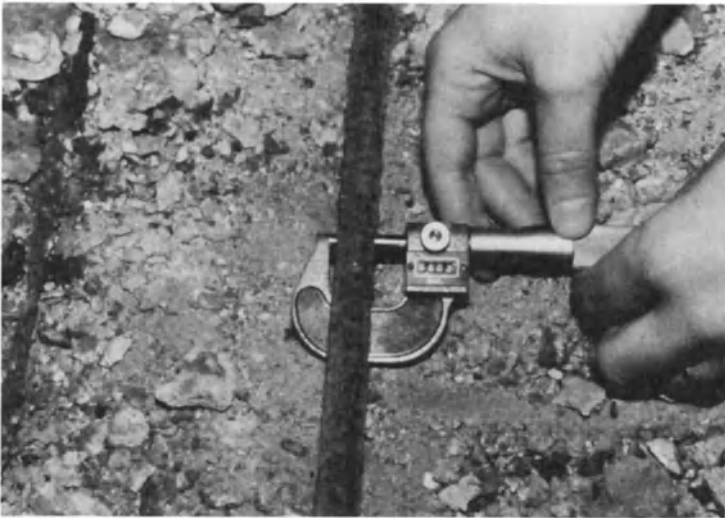
Figure 19-53: (b) Measuring extent of rebar corrosion.
