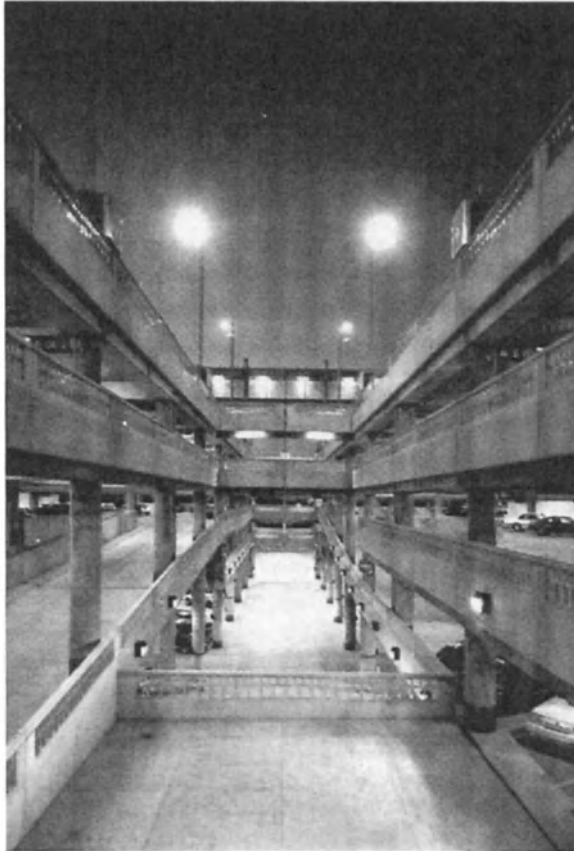
Figure 5-8. A light well acting as a court may be employed to meet requirements for distance from any point on a floor to an open side. Photo courtesy of Walker Parking Consultants.
