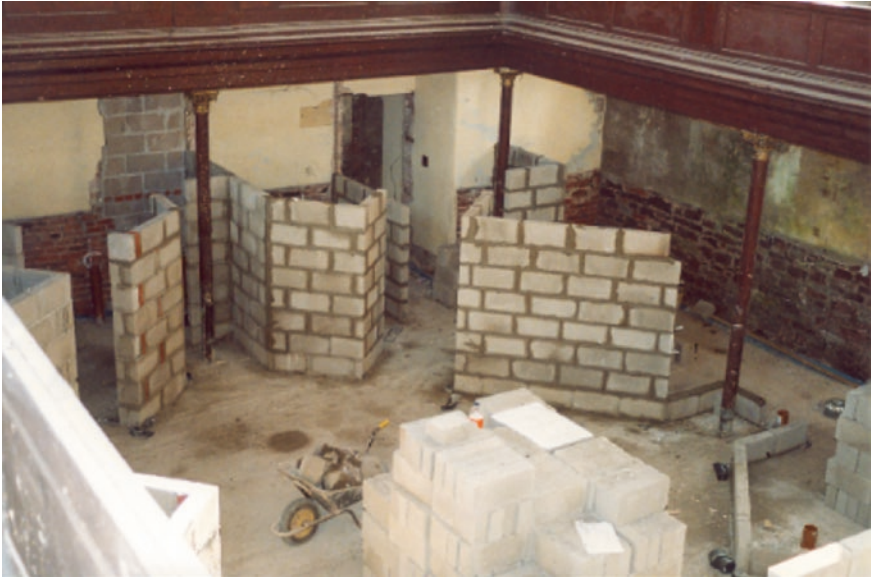
Fig. 4.10 Blockwork partitions before receiving plasterwork Glendower House Chapel conversion (Anthony Sully, designer of Glendower St Chapel conversion, Monmouth, Wales, 2002). Photograph by author
