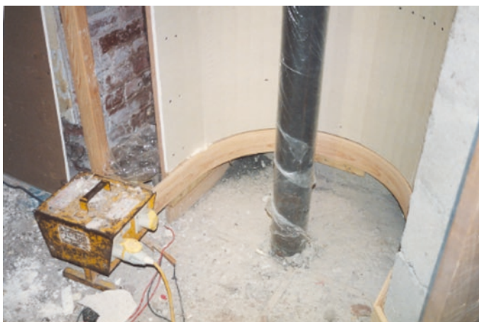
Fig. 4.12 Scored plasterboard to enable the curved plaster finish to be achieved. Photograph by author
