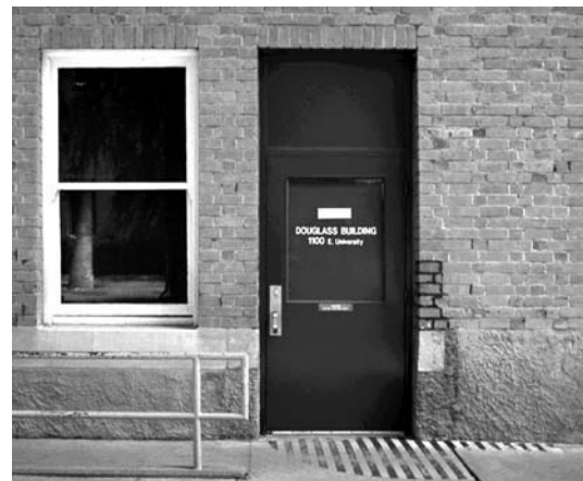
Figure 19.7 Door swinging into a walkway.
