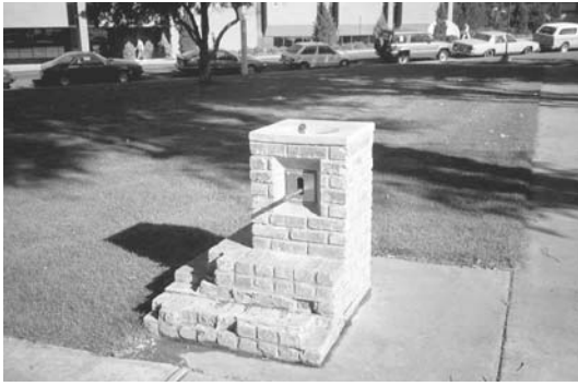
Figure 19.8 Abrasion on masonry steps.
